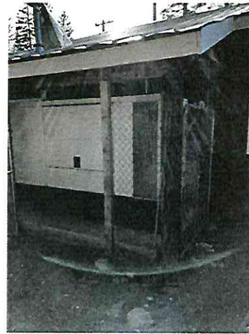
Figure 17 Backup power generator
