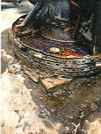
Figure 13 Pump 2 pedestal seal
