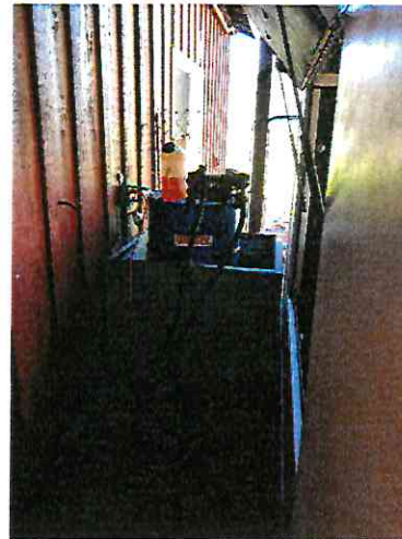
Figure 18 Backup generator fuel storage
