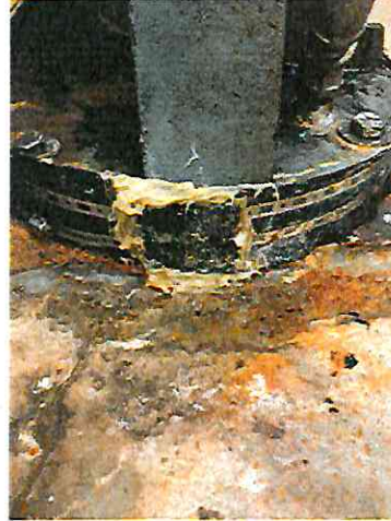
Figure 10 Pump 1 pedestal seal
